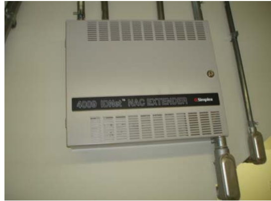
Photo 38. Fire Alarm System
