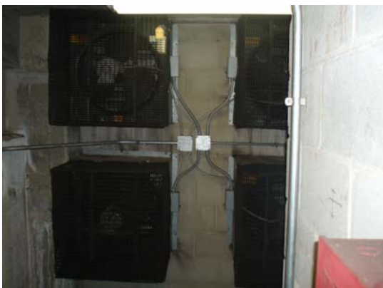
Photo 17. Elevator Exhaust Fans
