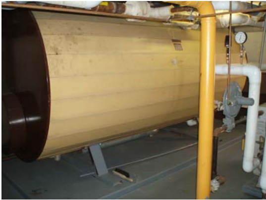
Photo 19. Hot Water Storage
