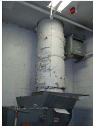
Photo 32. Chute at Compactor
