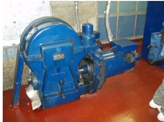
Photo 16. Elevator Motor and hoist
