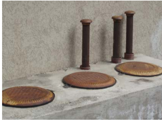
Photo 8. Fuel Fill Caps
