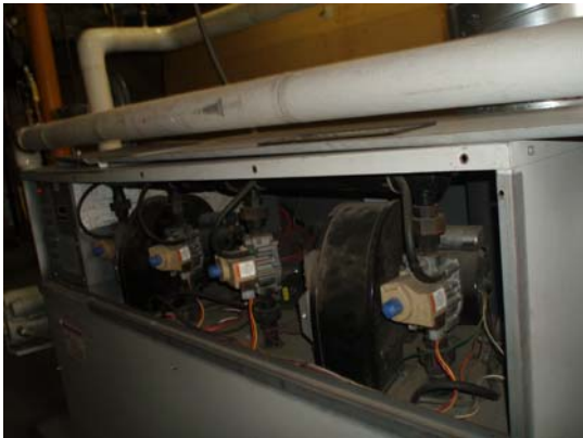
Photo 21. Boiler up close
