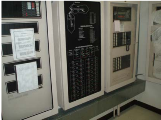
Photo 37. Fire Alarm System
